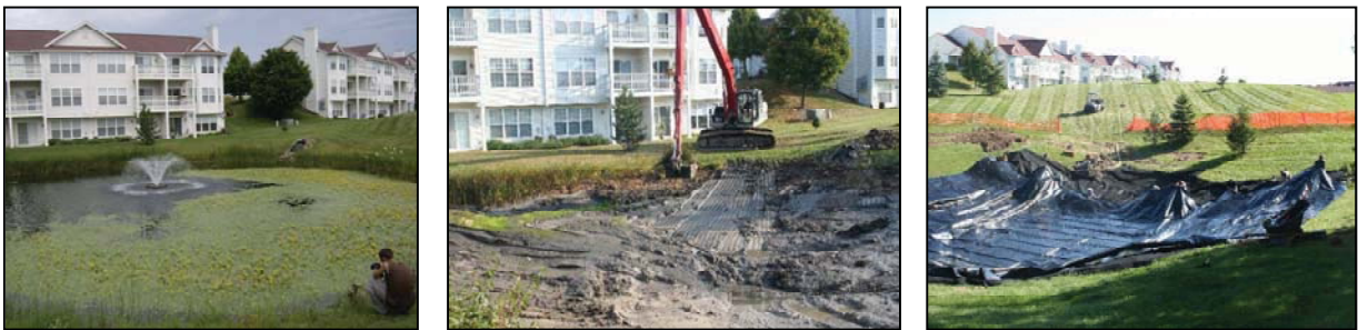
A Yellow Floating Heart infestation was discovered in two ponds in Walworth County in 2007. The ponds received multiple chemical treatments, were drained, dredged, lined, and final landscaping was completed in Spring of 2010. Total project costs exceeded $54,000 not including Walworth County and WDNR staff time. A few Yellow Floating Heart plants were found in September 2010 and were removed. The ponds continue to be monitored by the WDNR.
