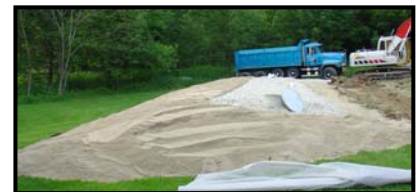
Washington County regulates private onsite wastewater treatment systems (POWTS) for any development that is not served by sanitary sewer.
