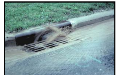
Chapter NR 216 of the Wisconsin Administrative Code is intended to reduce the discharge of pollutants carried by stormwater.
